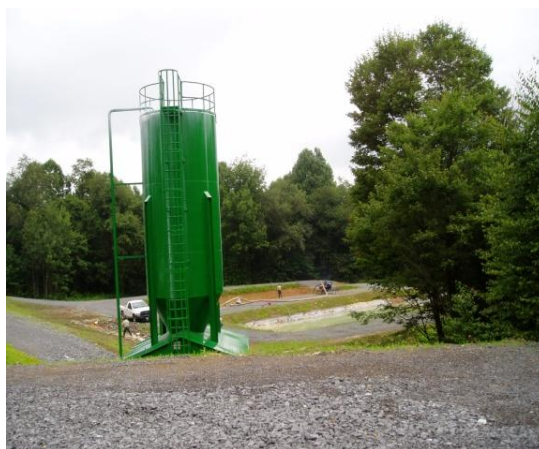
Treatment facility and settling ponds
