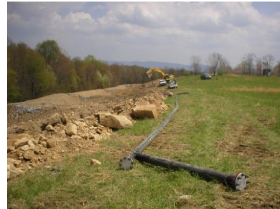
Sludge pumping line and sludge cells
